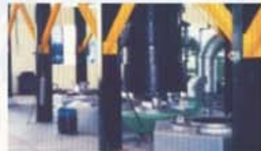
Fluidised Bed Plant for Dies
